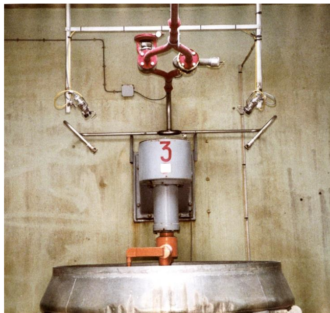
Fire suppression setup – Source Pyroalliance
